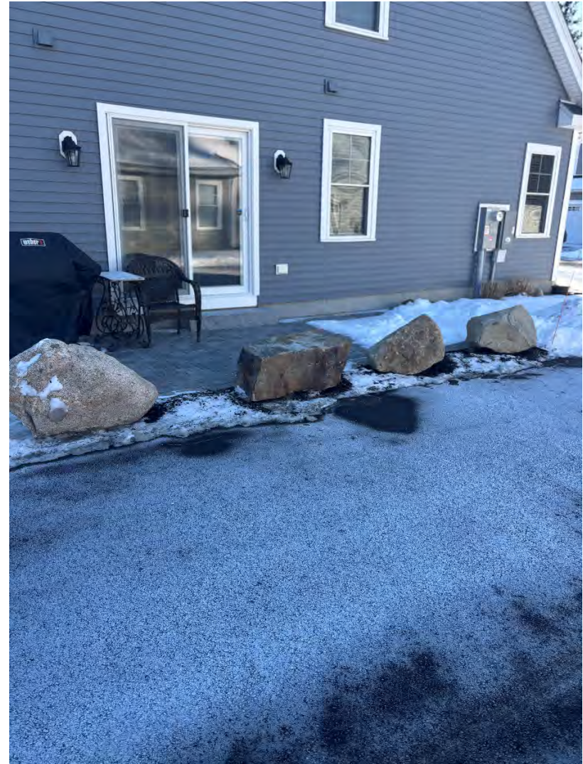
taken from: Izzys Lane, looking East Protective Boulders installed along Unit #15 Patio
