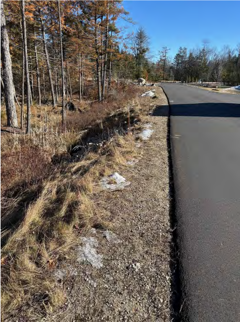
taken from: Fieldside Lane northern shoulder, looking East view of Side Slopes in vicinity of 36" CPP Wetland Crossing invert out, West of Izzys Lane intersection
